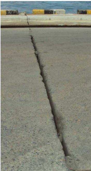
Figure 17-2: Gap at Corner Section
