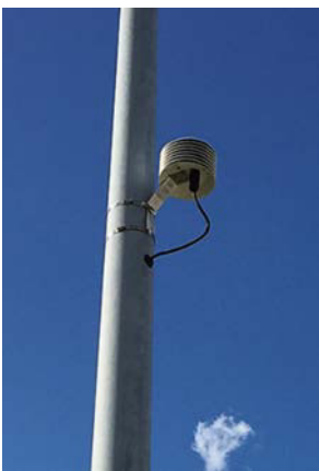
eNose mounted onto a lightpole.
